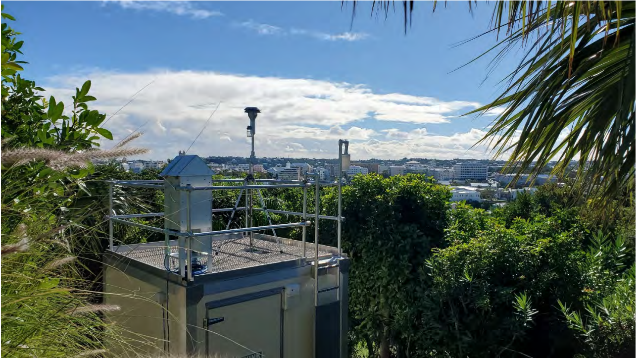
Figure 3 BDA2 Vegetation in Compliance From Parking Area
