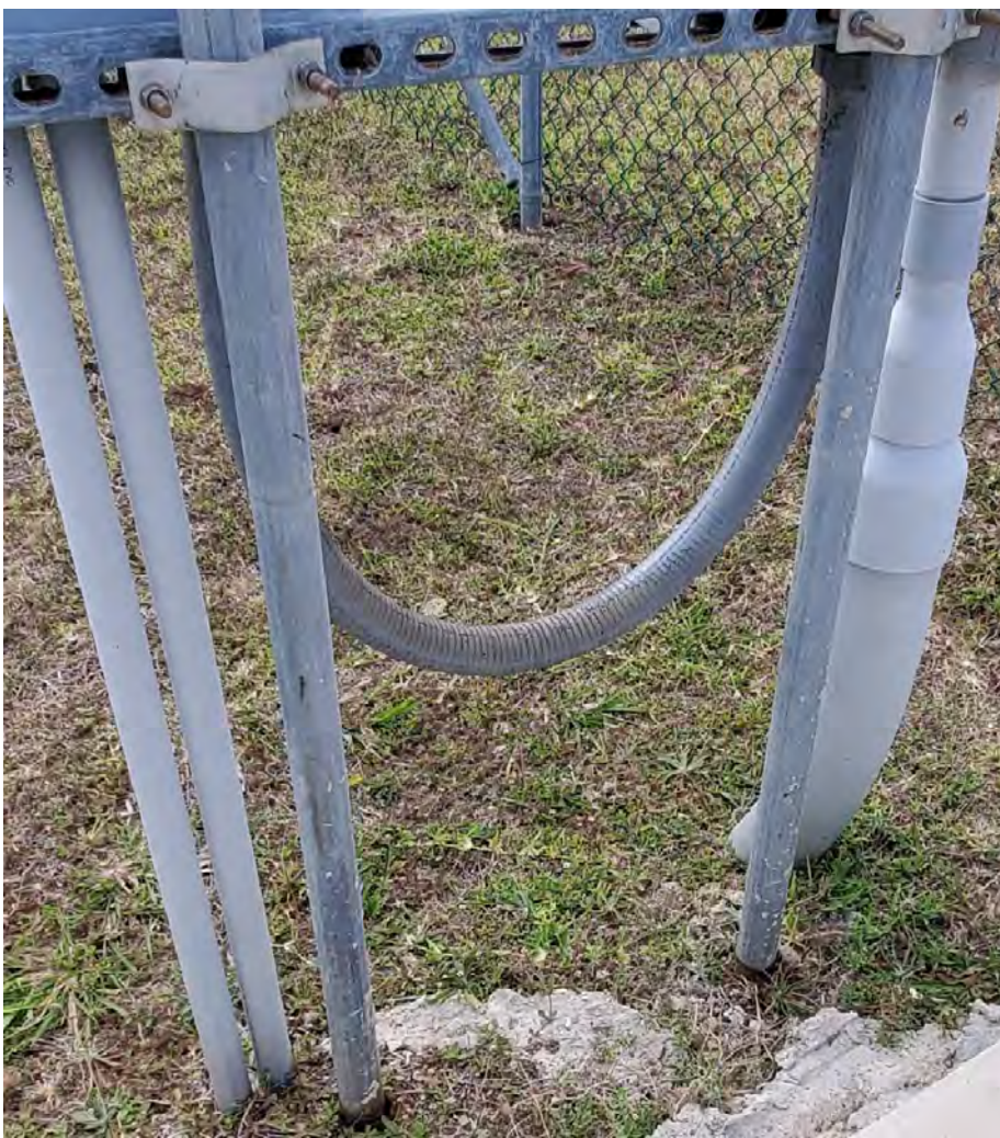
Figure 4 Potential Safety Hazard – BDA1 Electrical Panel
